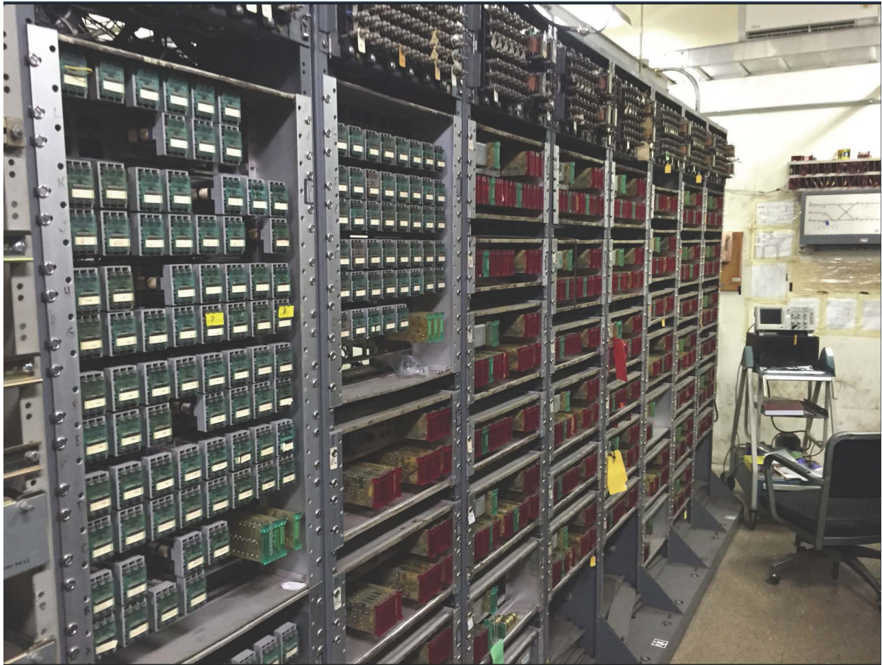
FIGURE 10: Red Line & Orange Line Signals: Existing Centralized Equipment Room with Analog Equipment
